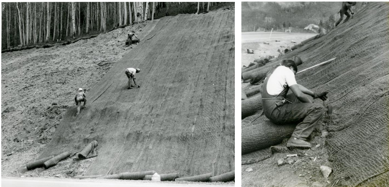
Figures 13 and 14. Placing jute netting on cleared slopes on Vail Pass to help stabilize and revegetate the slopes. 98
