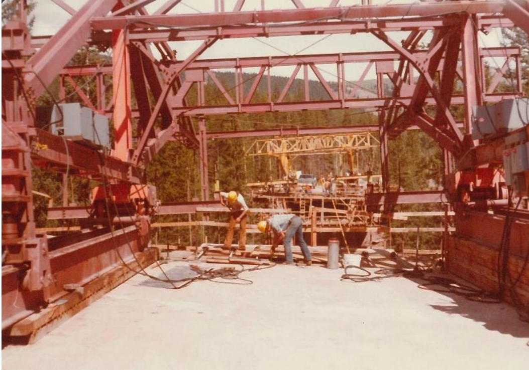
Figure 24. Miller Creek eastbound structure, with the form traveler and gantry for cast-in-place concrete box girder construction, September 1977. 124
