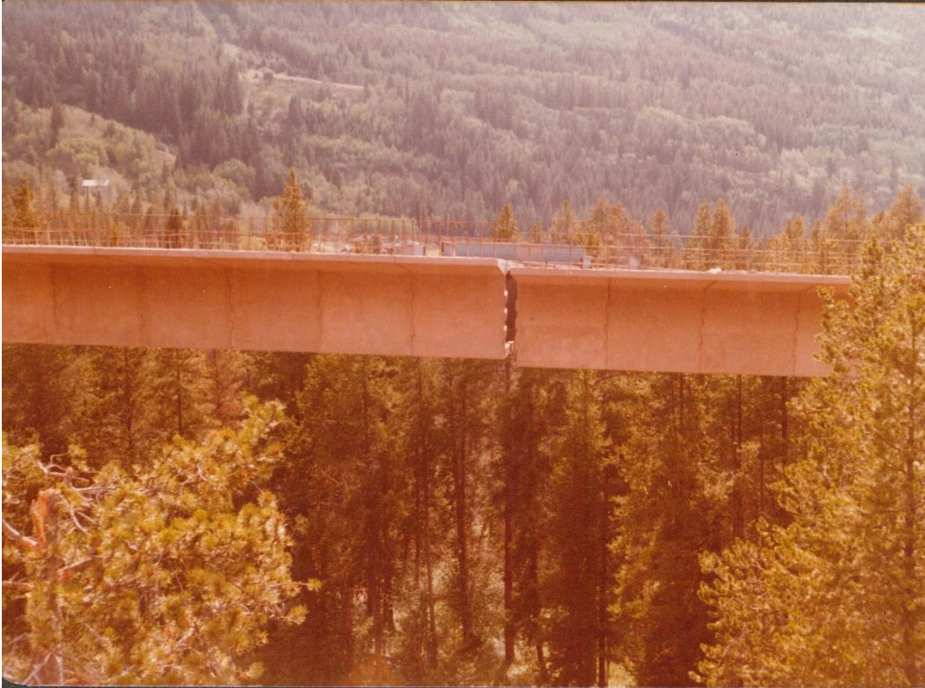
Figure 23. Gore Creek prior to the post-tensioning of the joint closure, westbound structure, August 5, 1977. 121
