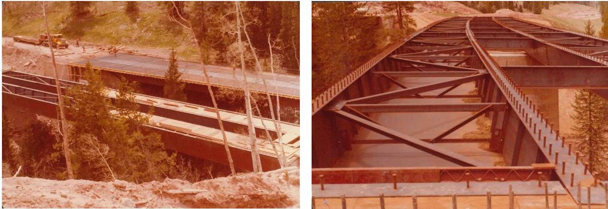
Figures 18 and 19. Welded steel box girder bridges under construction on Black Gore Creek, May 25, 1977. 108
