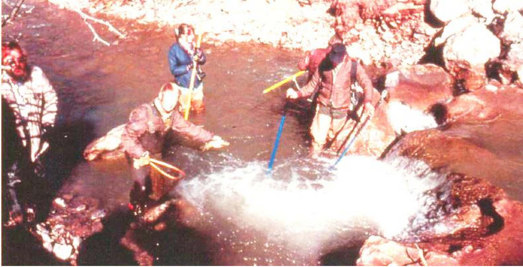
Figure 11. Biologists checking Tenmile Creek for trout habitat in a section rebuilt as part of Vail Pass I-70 construction. 90
